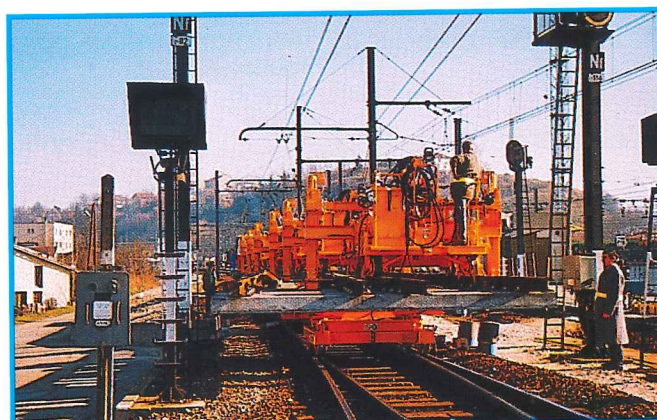
Travel through a station.
